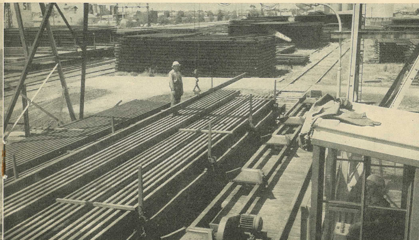
WELDED RAILS BEING LOADED ON A WAGON FOR THE STANDARD GAUGE TRACK
